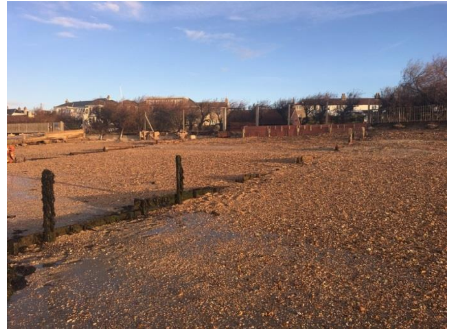
After FBC make-safe works
